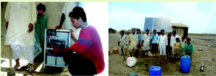
Solar energy panels installed in creek villages.
